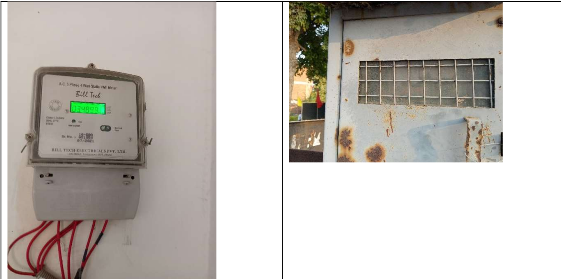
Fig 16: Electric meter photograph inside and outside the premises
