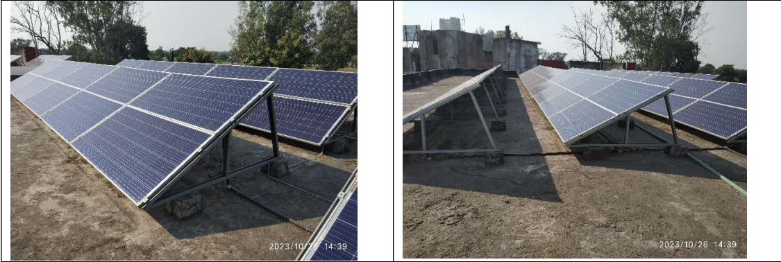
Fig 19: solar power plant on the roof top
