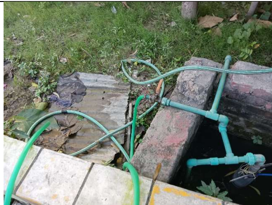
Fig 15: Water been extracted from the bore well
